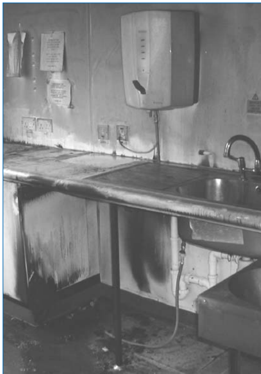
The damaged kitchen
